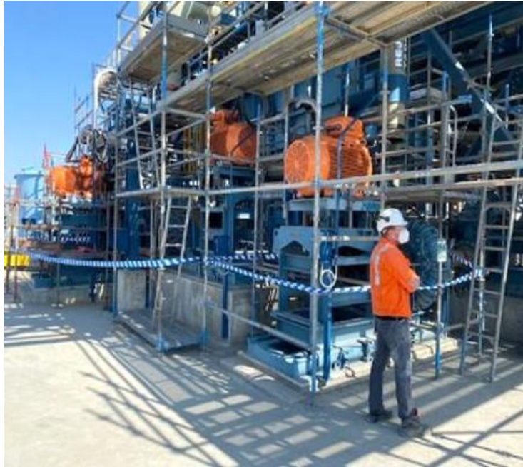
Cyclone energization and cold commissioning
