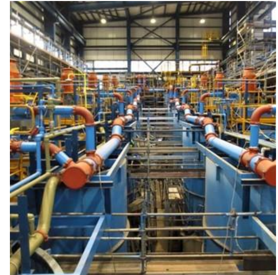
Flotation building piping
