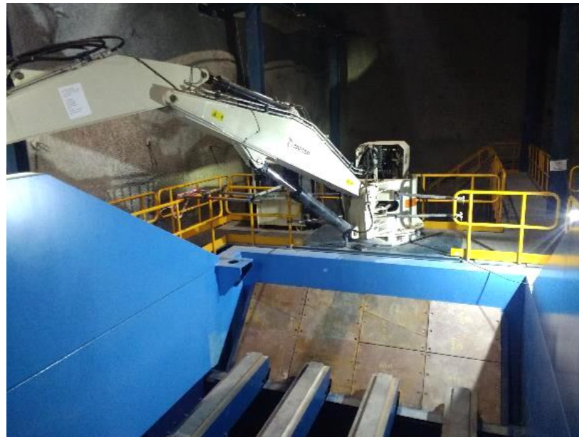
Crusher chamber – rock breaker and hopper
