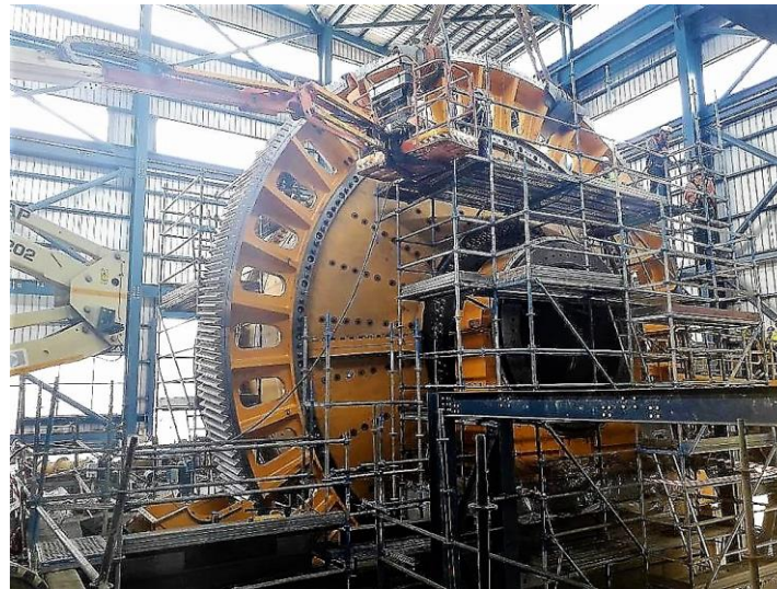
SAG mill gear ring installed
