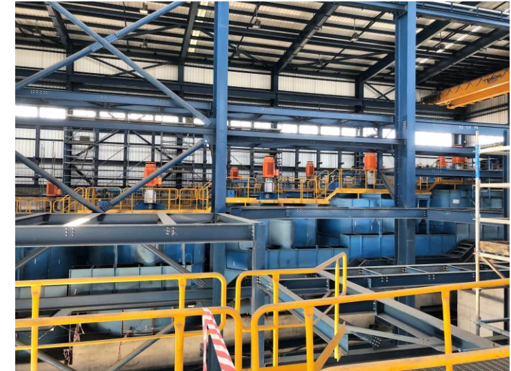
Flotation cells in new zinc plant building
