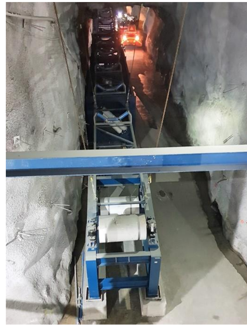
Turnover Station Conveyor #3
